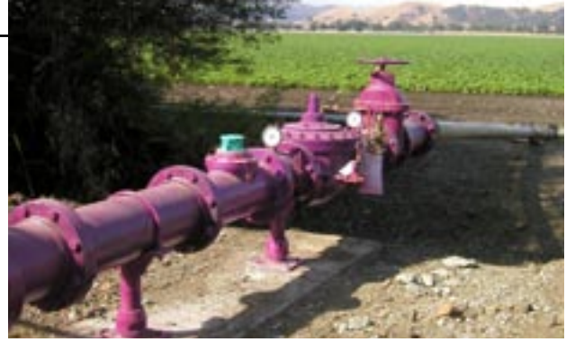
Recycled water pipeline
